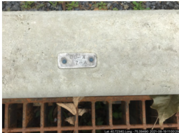
Photo #: 11 Outfall (Field)-003 Description: each stormwater inlet has a designation tag Photo taken by SCOTT CONFER
